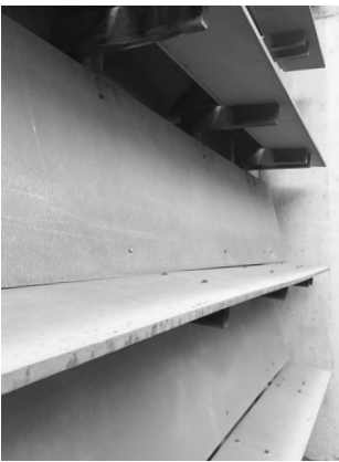
Fig. 14. Eternit plates assembled in the Storage Building.
